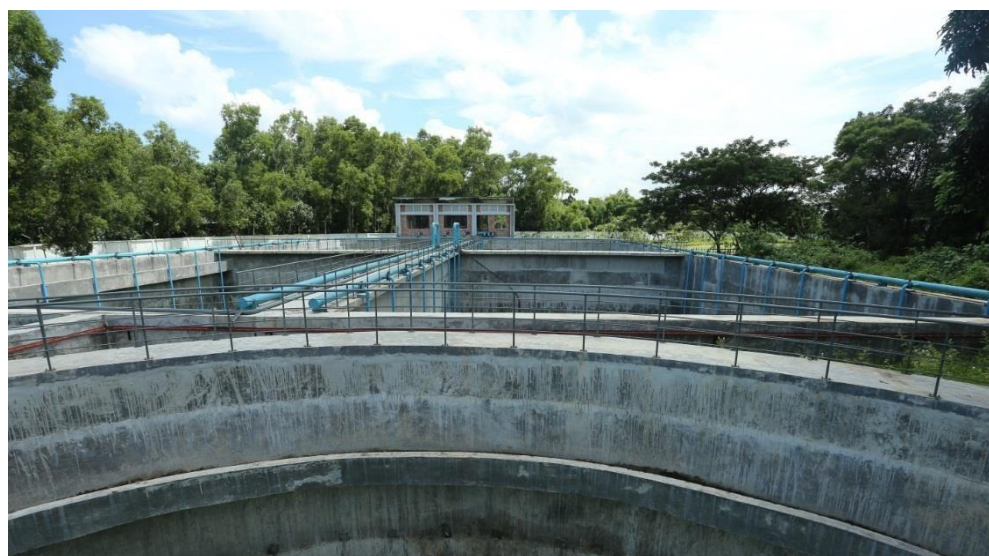
Figure: Complete Biological Effluent Treatment Plant 300 m 3 /hr
